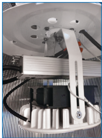
A retrofit LED lamp and driver installed inside a high-bay fixture
