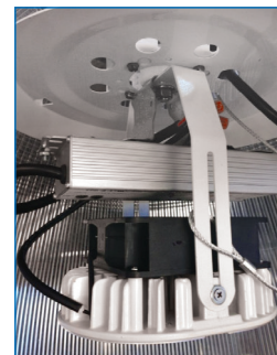
A retrofit LED lamp and driver installed inside a high-bay fixture
